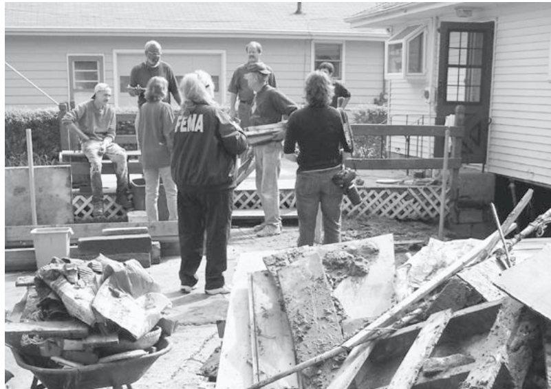
State and federal damage assessment officials speak with Highland residents whose basement wall collapsed from the mid-September flooding. FEMA Photo by Gene Romano
