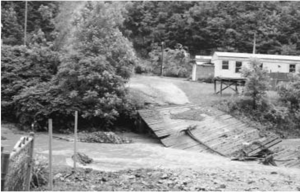
Floodwaters and landslides from the Memorial Day weekend storms washed out bridges and roadways in Mingo County, leaving many people temporarily stranded. Photo by West Virginia Office of Emergency Services
