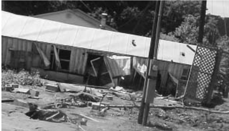
This mobile home in Mingo County was seriously damaged by the Memorial Day storms. Photo by West Virginia Office of Emergency Services.
