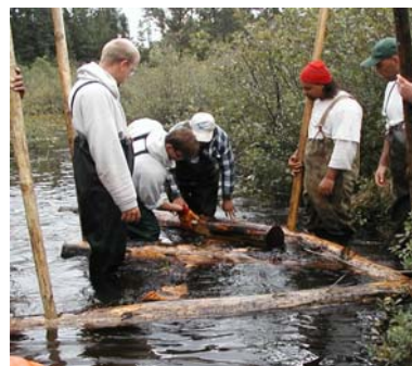
In-stream wooden structures were installed in shallow Ox Creek (Douglas County) that caused water to scour deep holes, providing fish habitat.
