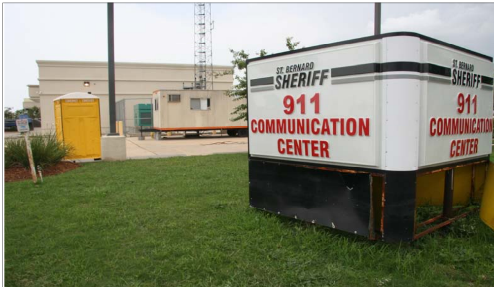
Chalmette, LA, -- Repairs are nearing completion at the St. Bernard 9-1-1 Center and operations are scheduled to resume in August 2008. FEMA funded the complete repair of the strategic communications center and related equipment, which suffered more than $1.1 million in damages. Barb Stumer/ FEMA photo
