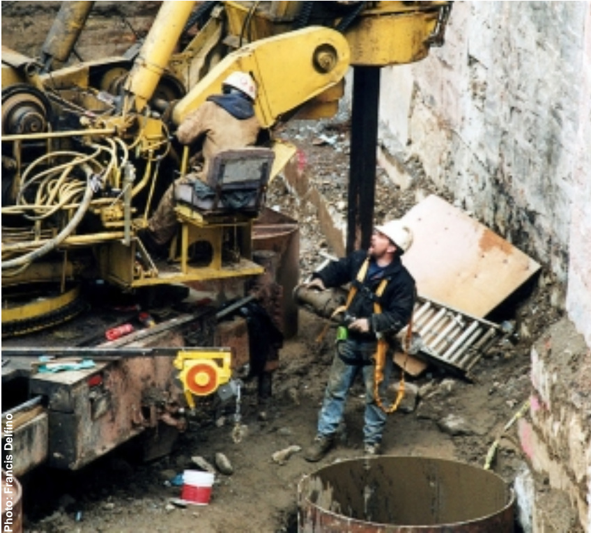
Workers drill holes in the foundation of Arvin Gym in preparation for pouring cement.
