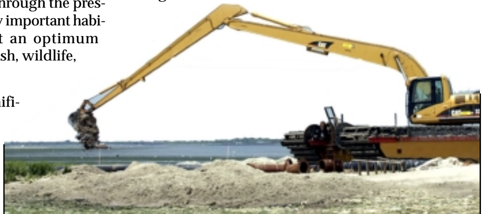
The restoration plan for Elders East and Elders West includes restoring the existing vegetated areas and the sheltered and exposed mudflats by placing fill material up to an elevation that is suitable for low marsh growth.
