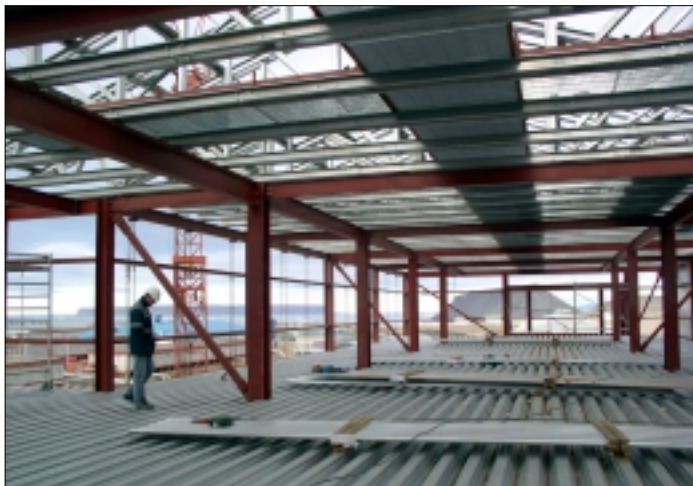
A contractor inspects the new flooring material during construction of the new dorm.
