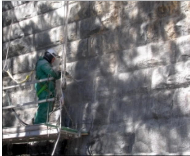
A worker uses small coarse grained silica under water pressure to clean the calcite build-up along the seams of the Lusk dam masonry stones.
