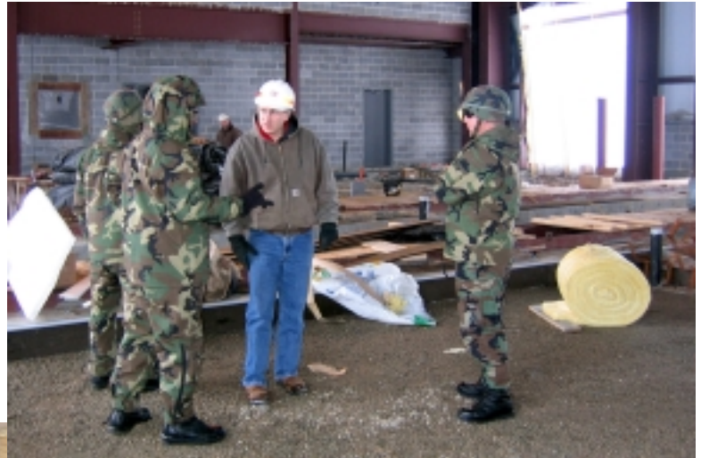
(Above) Soldiers from the 411th Engineering Brigade New York Army National Guard and Marty Tokos, project engineer, Fort Drum resident office inside one of the vehicle maintenance facilities at Fort Drum. The VMF 1 is a 33,000 square foot pre-engineered metal building which includes 9 vehicle service bays, 88 work bays and 5 administrative areas in two major buildings.
