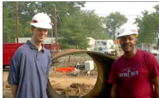
Christopher Myers (left) of Construction and Milton Ricks of Engineering at the Greenbrook flood control project. (below) The pipe has a 66 inch steel casing. The casing is then jacked by the tunnel boring machine before a 56 inch sewer line is placed inside.
