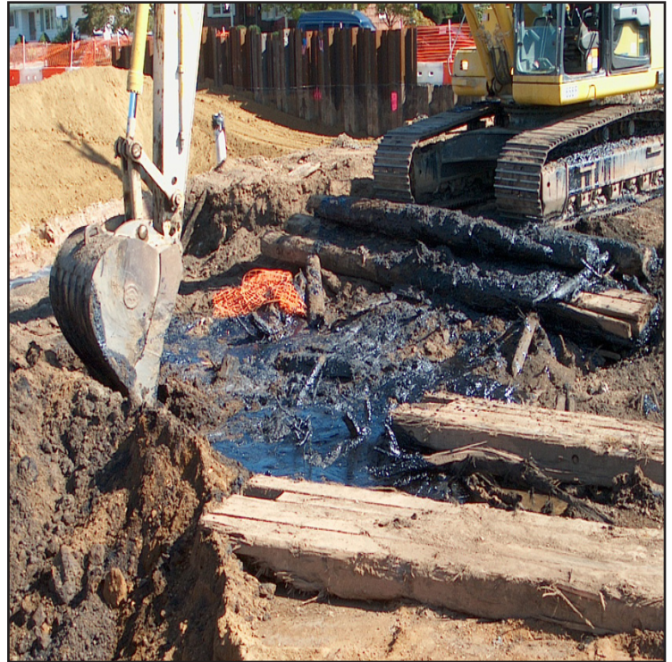
Contaminated soil was excavated from all residential properties in the Claremont Development containing high amounts of creosote.
