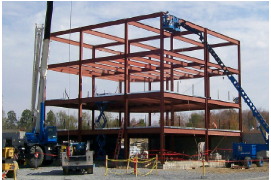
The 10100 barracks construction project at Fort Drum, N.Y. The complex is designed to house 238 Soldiers. Photo: Marty Tokos
