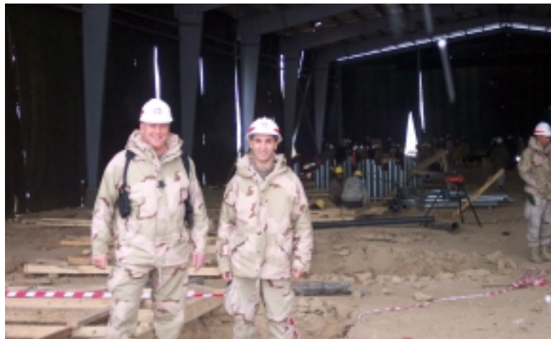
(l-r) Col. O'Dowd, District and Doug Liete inside a structure being refurbished in Afghanistan.
