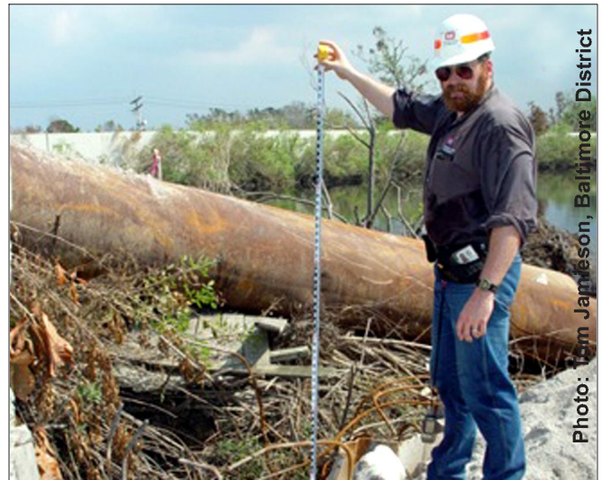
David N. Rackmales, P.E., structural engineer, Engineering Division, Design Branch, collects preliminary flood damage data on a failed section of the London Street Canal floodwall in New Orleans, La. Rackmales deployed to Louisiana in Sept. as part of a Forward Engineer Support Team in conjunction with North Atlantic Division's response to Hurricane Katrina.
