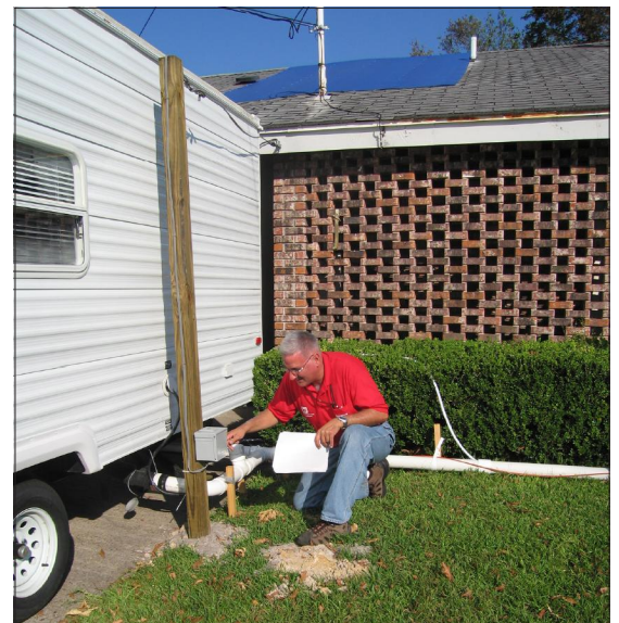
Randy Hintz, New York District quality assurance supervisor, Operations, checks out the electrical installation on a travel trailer on private property.
