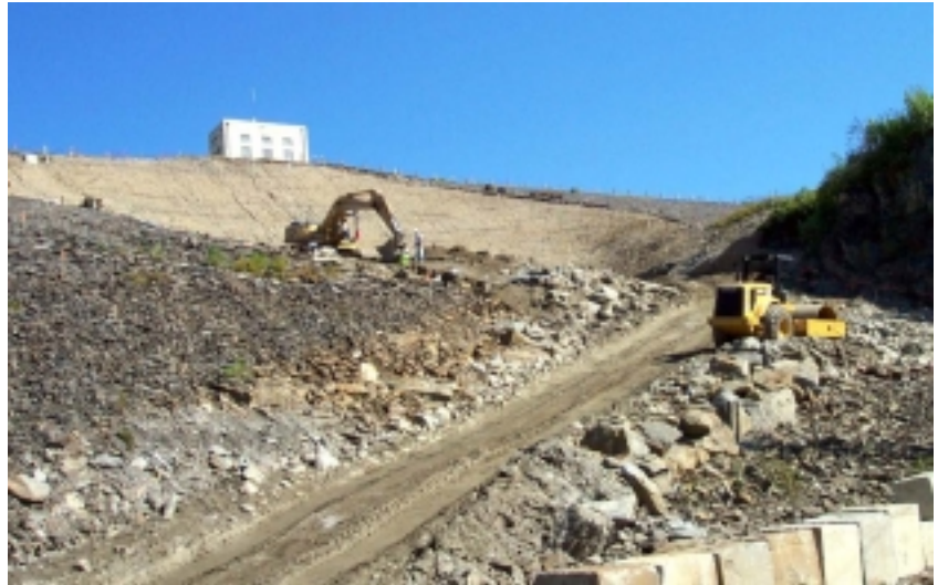
Bulldozers excavate along the toe of the dam as backfill placement is also necessary at the shell zone following placement of filler material.
