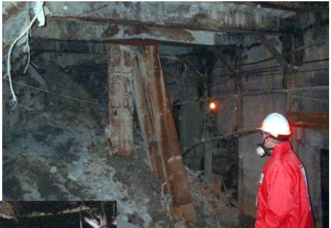
Inside the subway train tunnel, Randy Hintz of Emergency Operations observes the huge amount of structural damage underneath the World Trade Center site. Collapsed building columns from the skyscrapers penetrated the subway tunnel beneath the ground.
