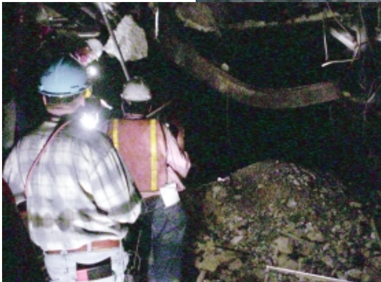
Inspectors examine the damage in the subway tunnel below the World Trade Center.
