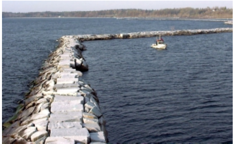
The Burlington Breakwater is comprised of rock-filled timber cribs capped with concrete or rock on a rubble mound.
