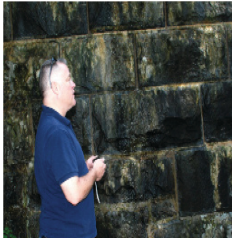
Marty Goff, dam safety specialist with New York District, examines a wet spot on the Lusk Dam at West Point. He regularly checks dams at the installation for signs of potential trouble, such as the wet spots above. Photo Credit: Christopher Gardner
