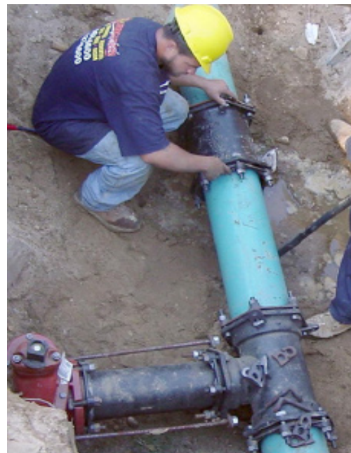
The Army Corps is replacing over 30 8-inch valves, installing a new irrigation system.
