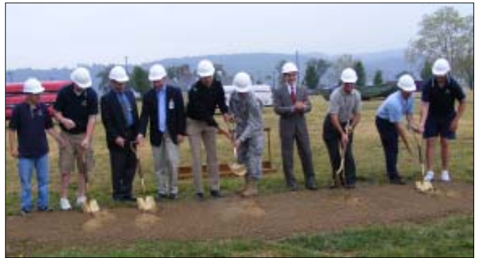
Navy Capt. Jim Naber (fifth from left), Col. Peter W. Mueller (center) and Defense Distribution Depot Susquehanna Pa., leaders and partners, turn the first shovel full of dirt to begin construction of the DDSP physical fitness center Aug. 29.
