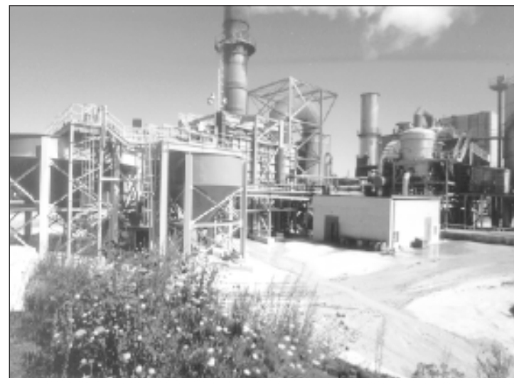
▲ The Passamaquoddy Technology Recovery Scrubber™ became a permanent part of the Dragon Products facility at the project's end.
