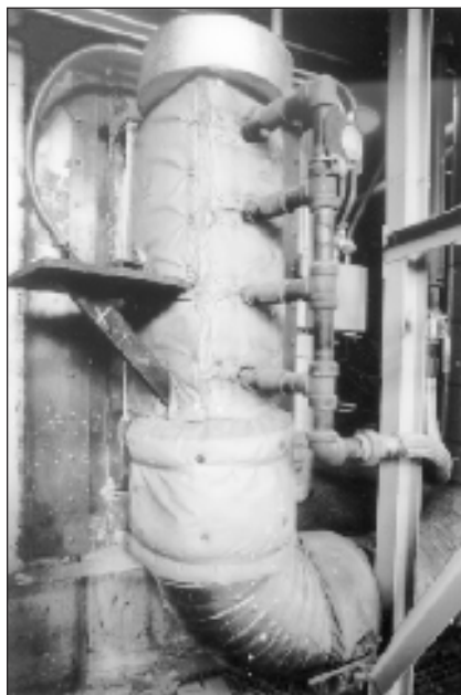
▲ The natural gas injector was installed on the corner of Hennepin Station's tangentially-fired boiler.
