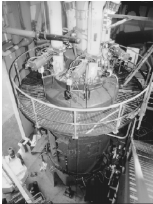
▲ The coal pulverizer is part of Babcock & Wilcox Coal Reburn. This system has been retained by Wisconsin Power and Light for NO x emission control at the Nelson Dewey Station.
