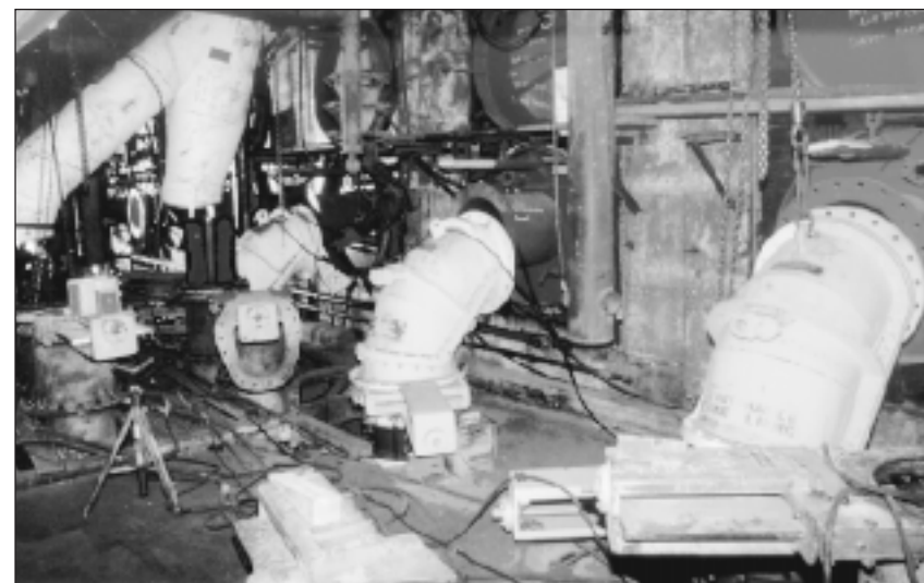
▲ The connections to the LNCB ® are viewed from outside the boiler.
