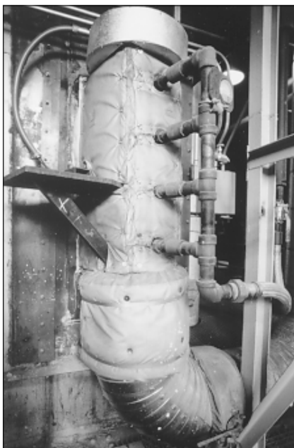
▲ The natural gas injector was installed on the corner of Hennepin Station's tangentially fired boiler.
