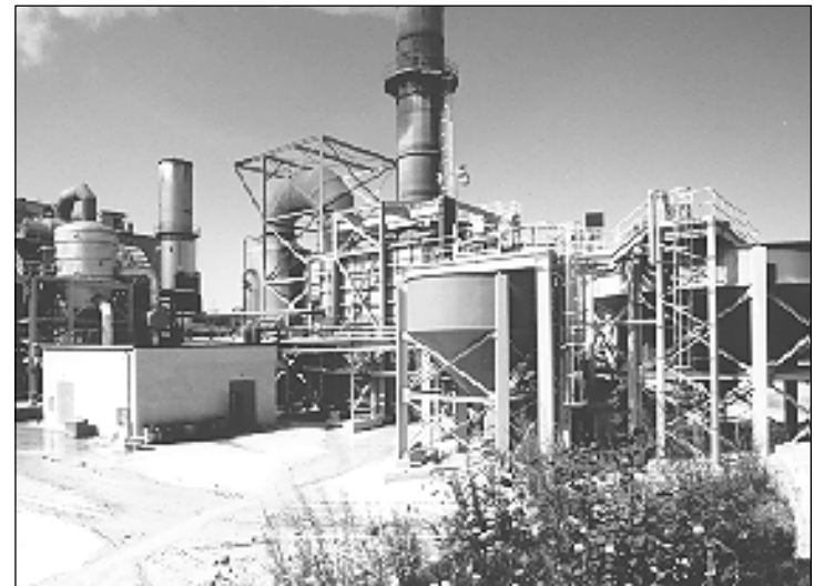
▲ The Passamaquoddy Technology Recovery Scrubber™ became a permanent part of the Dragon Products facility at the project's end.
