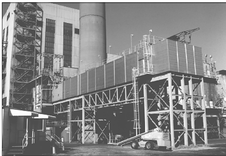
▲ Bechtel's demonstration showed that 50% SO 2 removal efficiency was possible using CZD/FGD technology. The extended duct into which lime slurry was injected is in the foreground.
