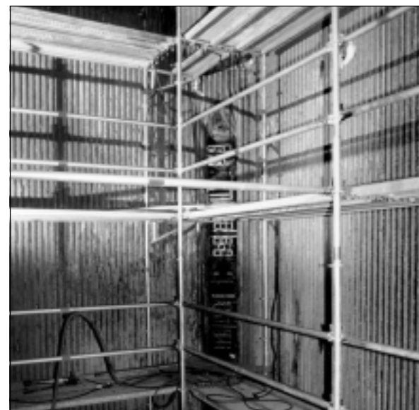
▲ A portion of ABB Combustion Engineering's Low-NO x Concentric Firing System (LNCFS™) is shown being installed on a tangentially fired boiler.
