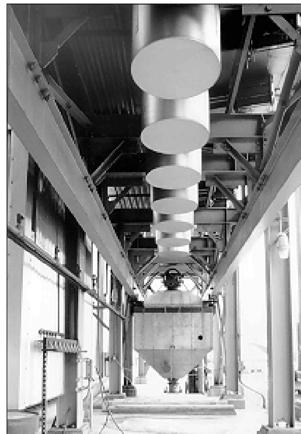
▲ The bottom portion of the SO 2 converter catalyst, with the catalyst dust collector hopper mounted on steel rails (center), is shown.
