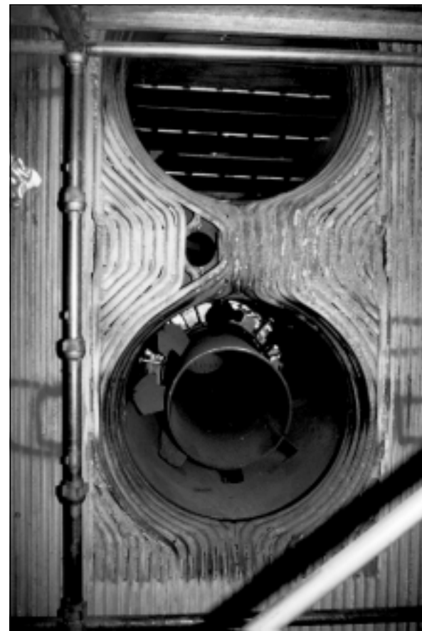
▲ The LNCB® is viewed from within the boiler.
