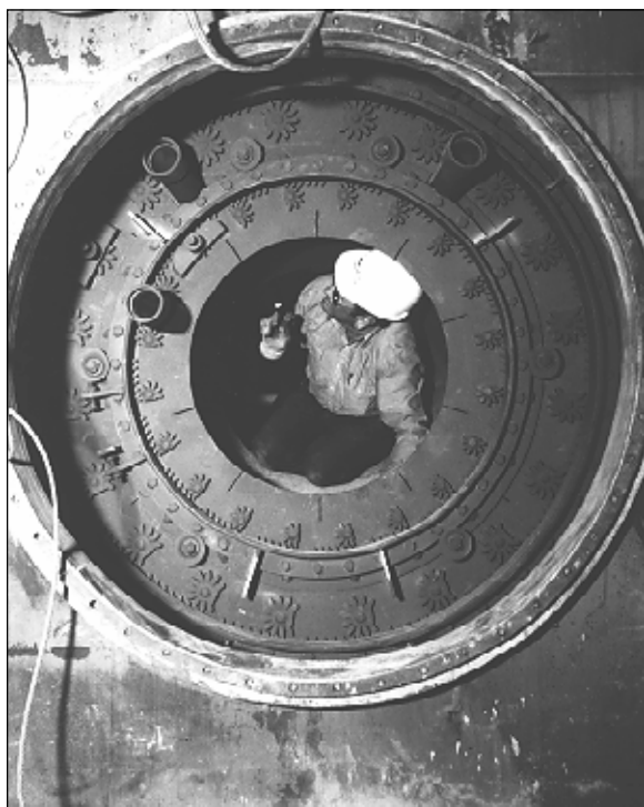
▲ A worker inspects the support ring for the Foster Wheeler low-NO x burner installed in the boiler wall.
