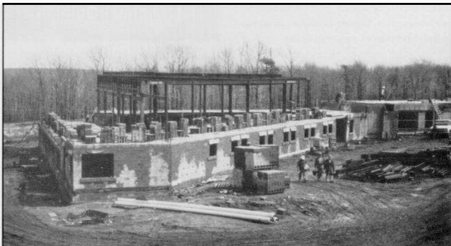
“...The amount of money being invested in prison construction and in the management of prisoners is overwhelming the taxpayers.” The Federal Correctional Institution at Minersville, Pennsylvania, currently under construction.
