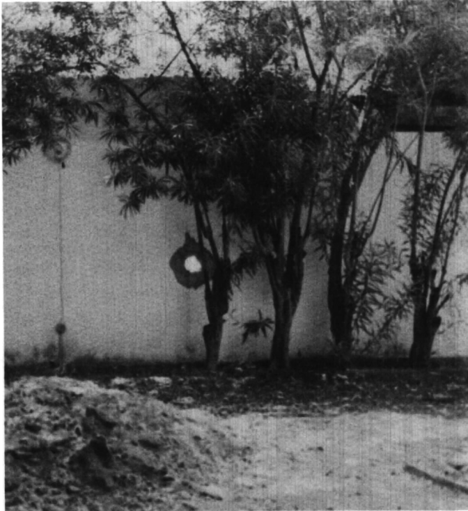
A rocket-propelled grenade was inadvertently fired through the perimeter wall of a U.S. Government residence in N'Djamena, Chad.
