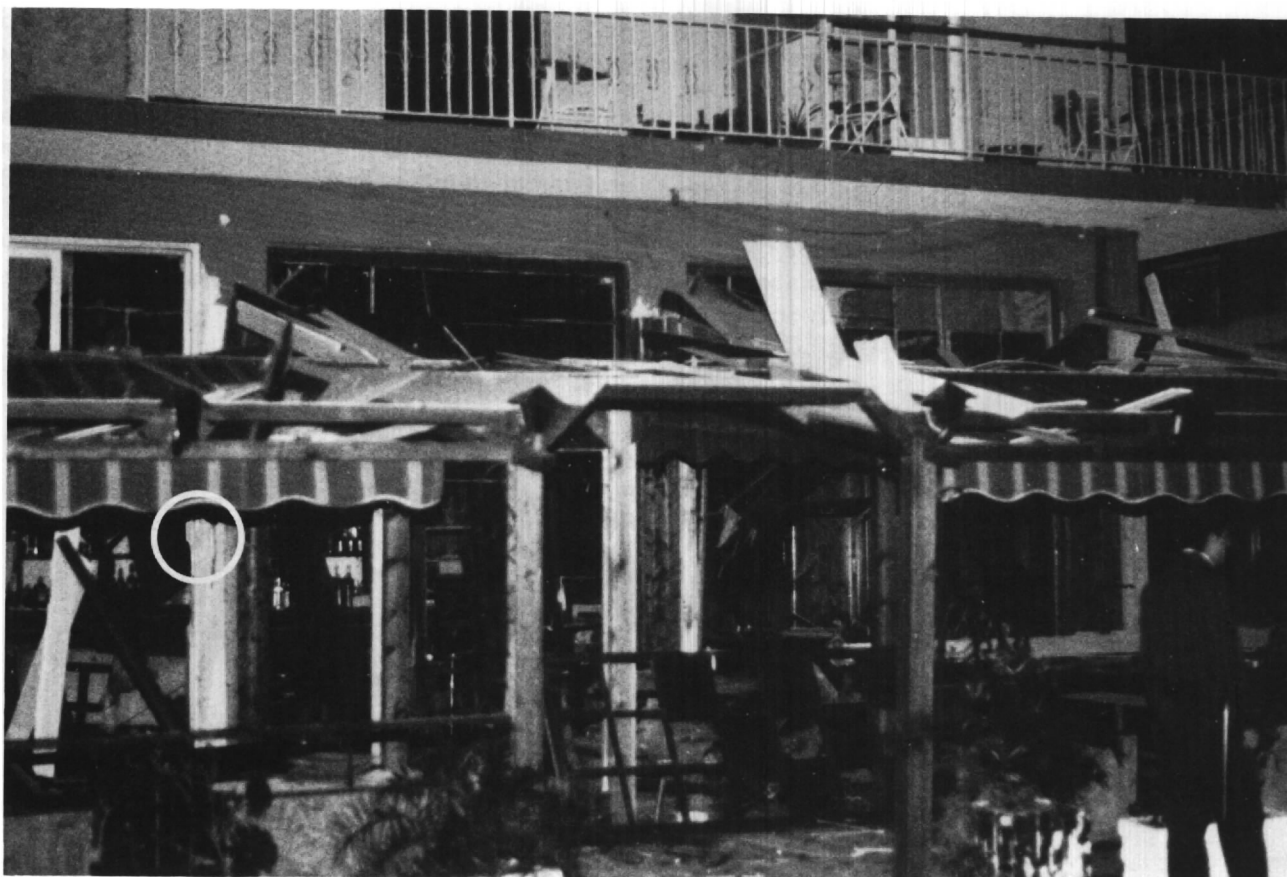
A bomb exploded causing extensive damage to Oscar's Pub and injuring 14 people (5 of whom were Americans). The circle indicates where the bomb was placed in a jacket that was hung near the entrance to the bar.
