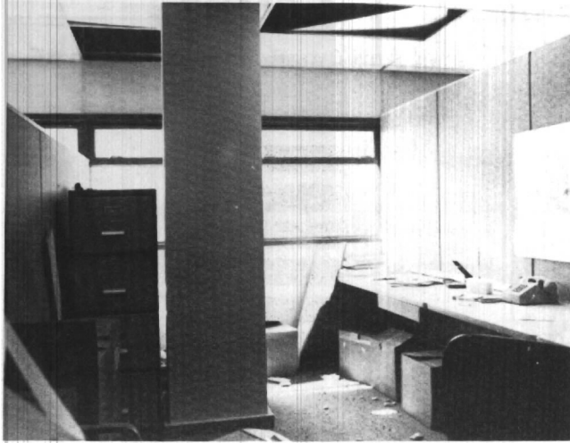
USAID office is damaged by the rocket.
