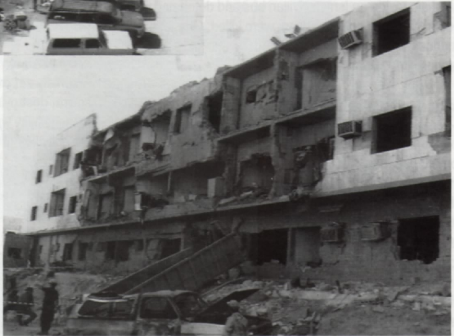
After the blast of the OPM/SANG building in Riyadh, Saudi Arabia.
