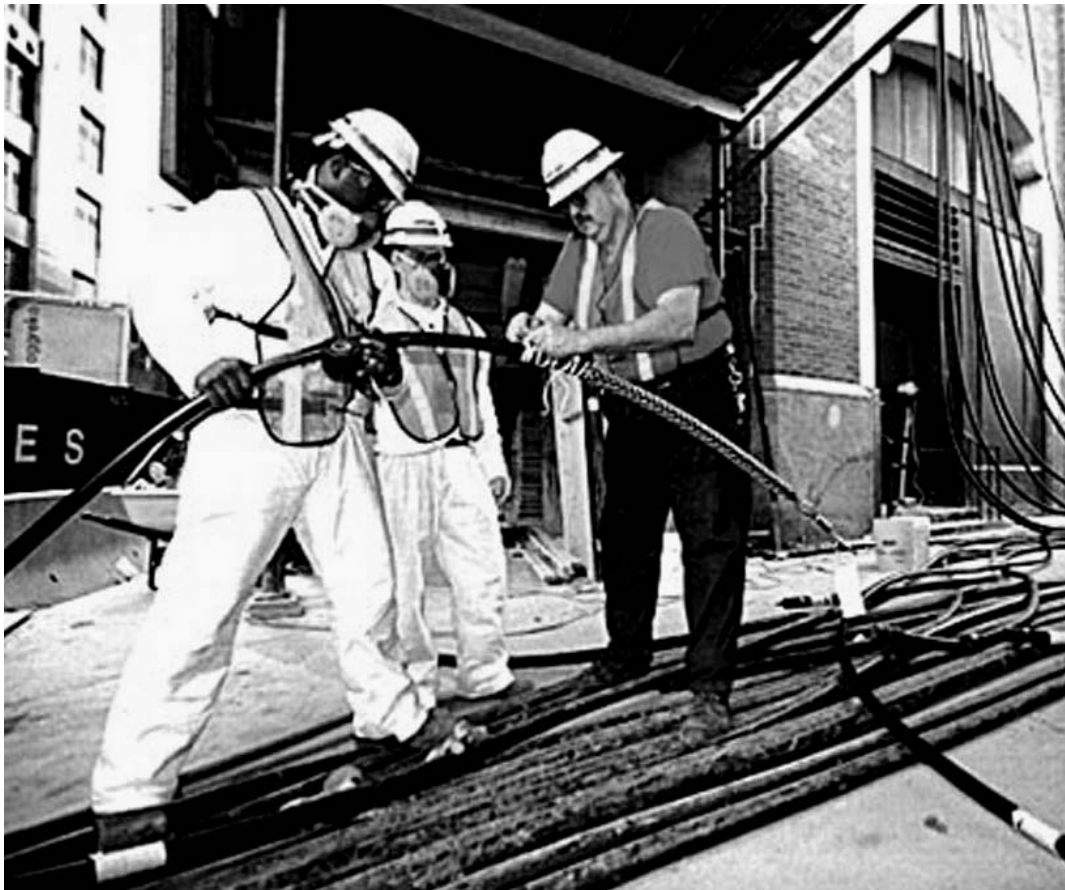
Verizon Communications technicians splice severed wire pairs in their efforts to restore communications in Lower Manhattan following the September 11 terrorist attack on the World Trade Center. (Photo courtesy of the Federal Communications Commission.)
