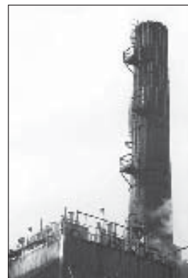
News of the ORNL Steam Plant's conversion to a state-of-the-art biomass-fueled boiler comes in the facility's 60th year of service. It came on-line in 1948.
