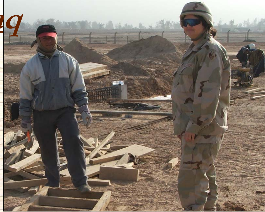
Billie Guille oversees the construction of concrete forms at her project in northern Iraq. (Photos provided by GRN)
