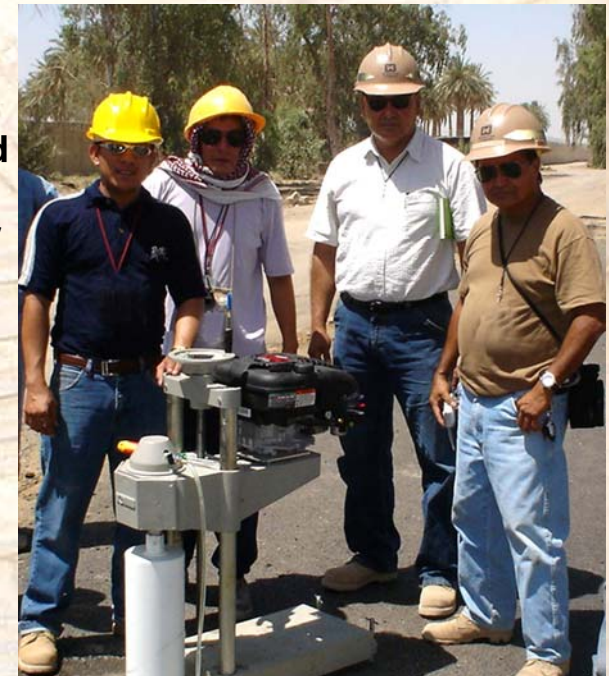
Wayne Birgado (right, in brown hard hat) and crew take a project road core sample.
