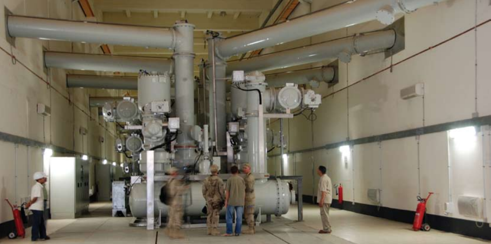
Gulf Region Division, al Rasheed substation personnel and the Siemens commissioning engineer talk about bringing the substation online in the 400kV Gas Insulated Switchgear building.
