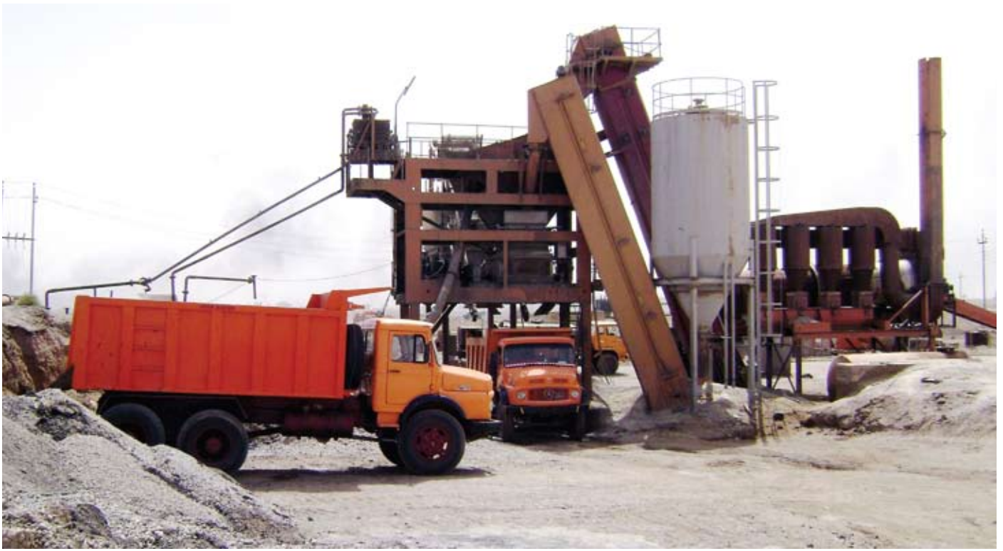
Turning out up to 80 metric tons of asphalt per hour, the Amarah asphalt plant is improving Maysan's roads.
