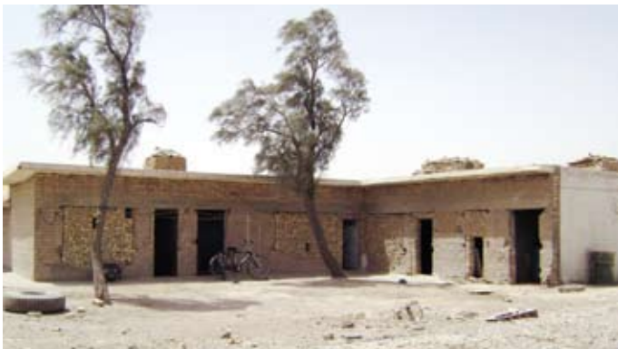
Before: The administration and site office facility prior to recently completed renovations.
