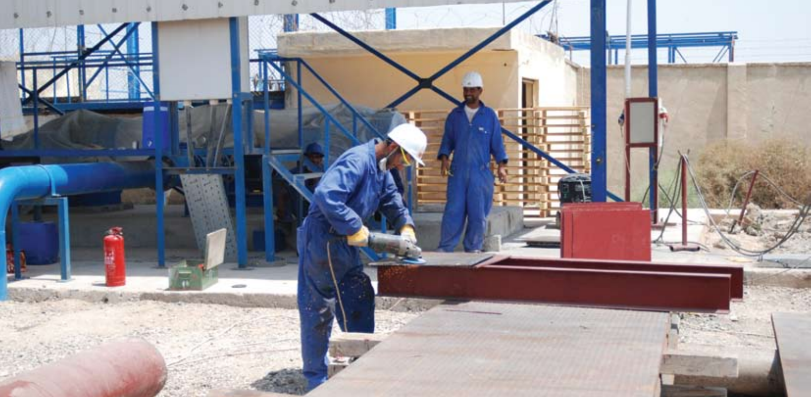
An Iraqi worker prepares to weld plate for a steel intake structure in the Shatt Al-Arab.
