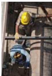
Overhead view from the tank catwalks of ongoing pipe welding work at Victory Base Complex's waste water treatment plant, see page 9
