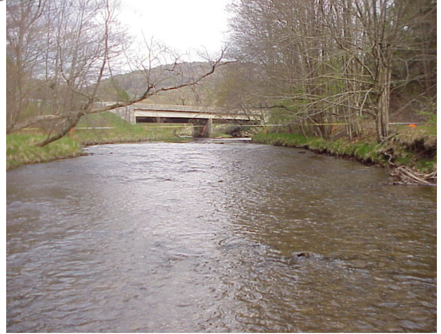
View looking upstream at the reach of Kinzua Creek containing cross section at station 730, May 8, 2003.
