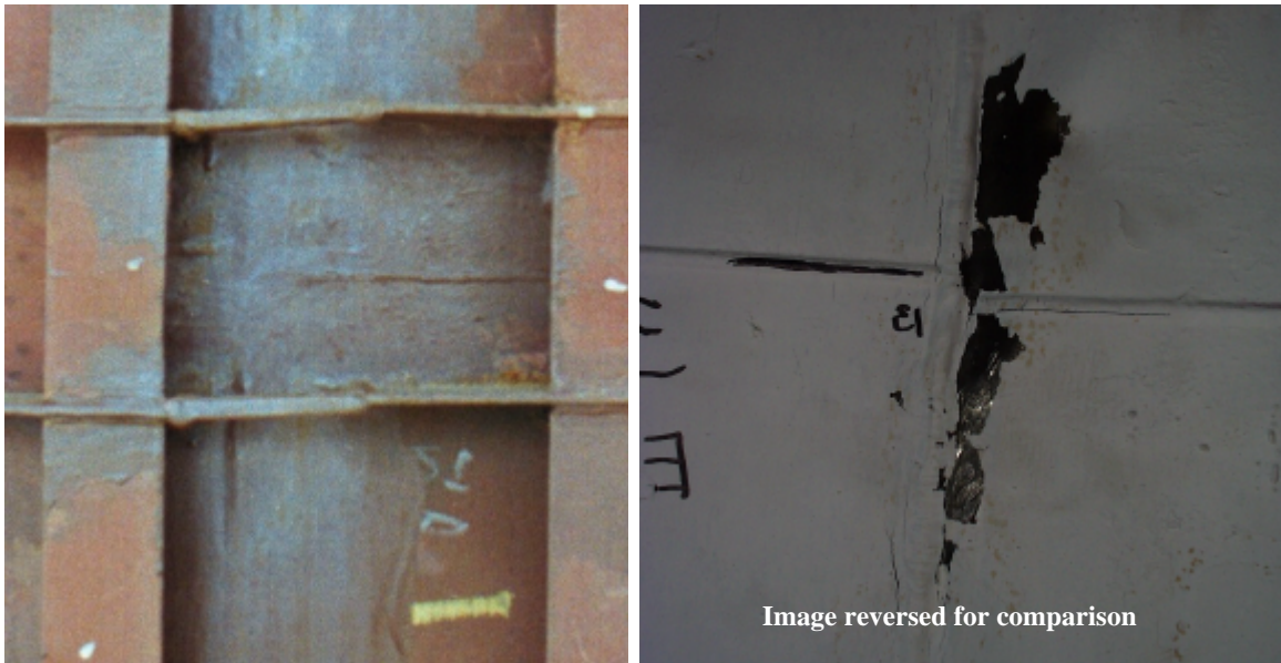
Figure 5.82 Tear #13 at E/H
