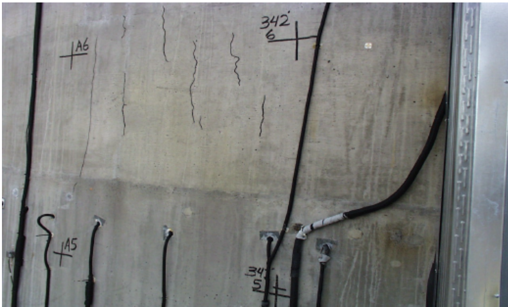
Figure 5.10 Pre-SIT Cracks at Azimuth. 350 degrees, Elev. 4680 to 6200 (Grid 45)
