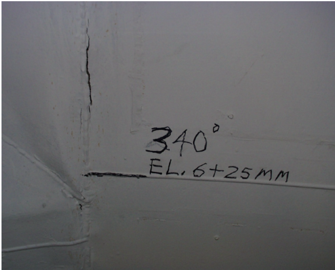
Figure 5.47 Liner Tear (#15) at E/H
