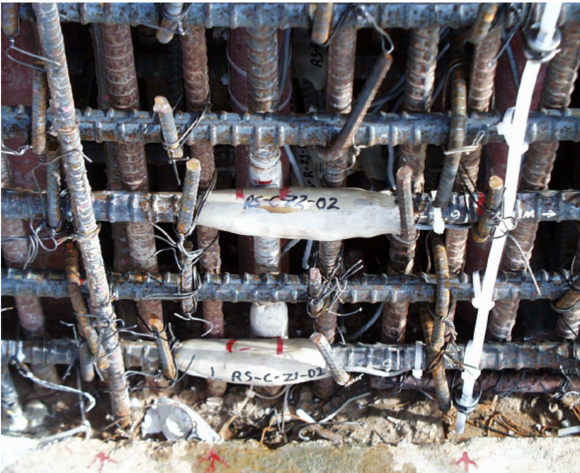
Figure 3.7 Rebar Strain Gages Installed in PCCV Model (Note SOFO Fiber Optic Concrete Strain Gage at right)
