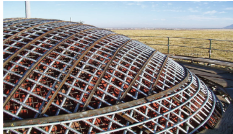
Figure 2.43 Dome Tendon Sheaths and Support Frame
