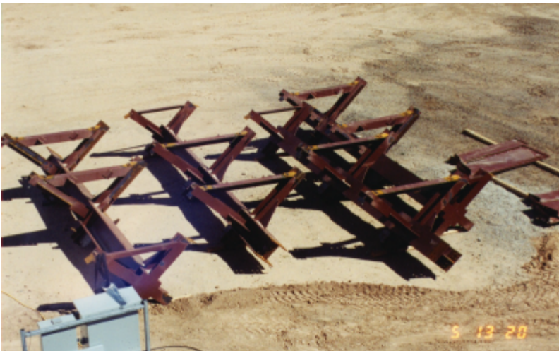
Figure 2.30 Instrumentation Frame Column 'Trees'
