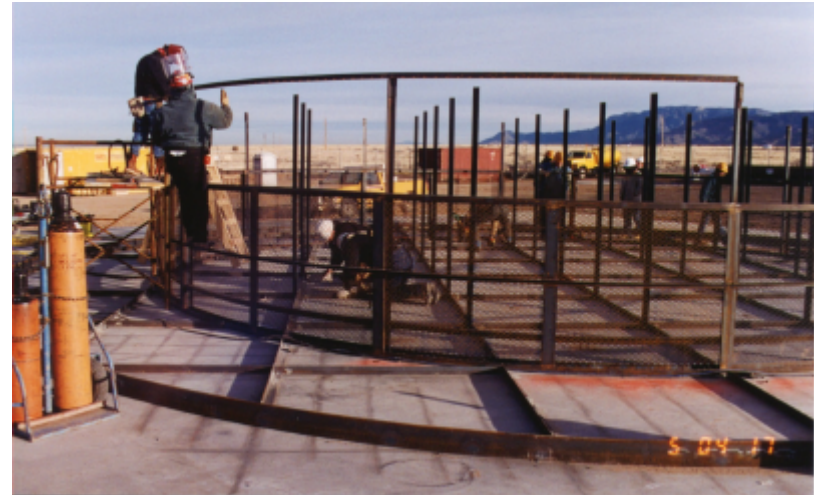
Figure 2.13 Basemat Rebar Support Frame
