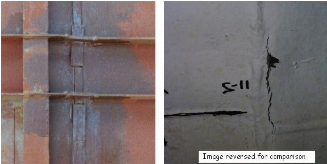
Figure 6. Photographs showing region of tear #11-2 from outside of liner (left) (prior to concrete placement) and inside of liner (right) (prior to removal of paint). Tear #11-1 was along the same vertical weld, but distant from the horizontal weld and associated horizontal stiffeners. Tears #11-1 and 11-2 were along the same vertical weld as tears #6-1 and 6-2.
