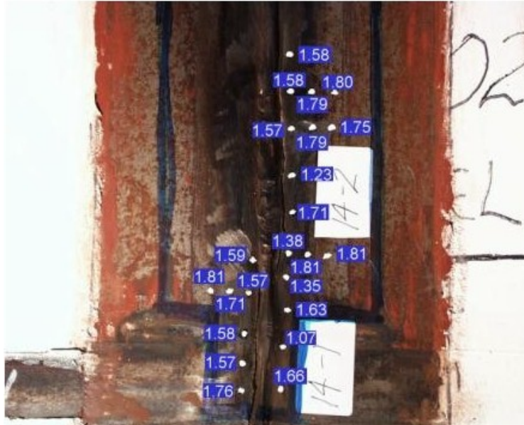
Figure 29. Liner thicknesses (in millimeters) measured ultrasonically in the vicinity of tear #14 (14-1 and 14-2).
