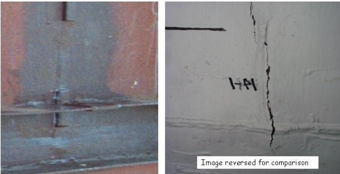
Figure 10. Photographs showing region of tear #14-1 from outside of liner (left) (prior to concrete placement) and inside of liner (right) (prior to removal of paint). Note missing segments of back-up bar in vicinity of repair weld and tear.
