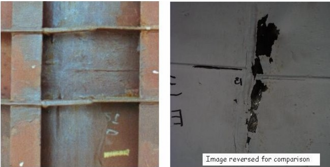
Figure 18. Photographs showing region of tear #13 from outside of liner (left) (prior to concrete placement) and inside of liner (right) (prior to removal of paint).
