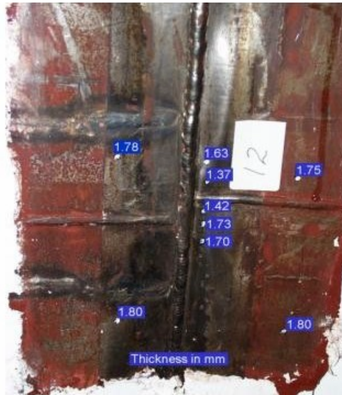
Figure 34. Liner thicknesses (in millimeters) measured ultrasonically in the vicinity of tear #12.
