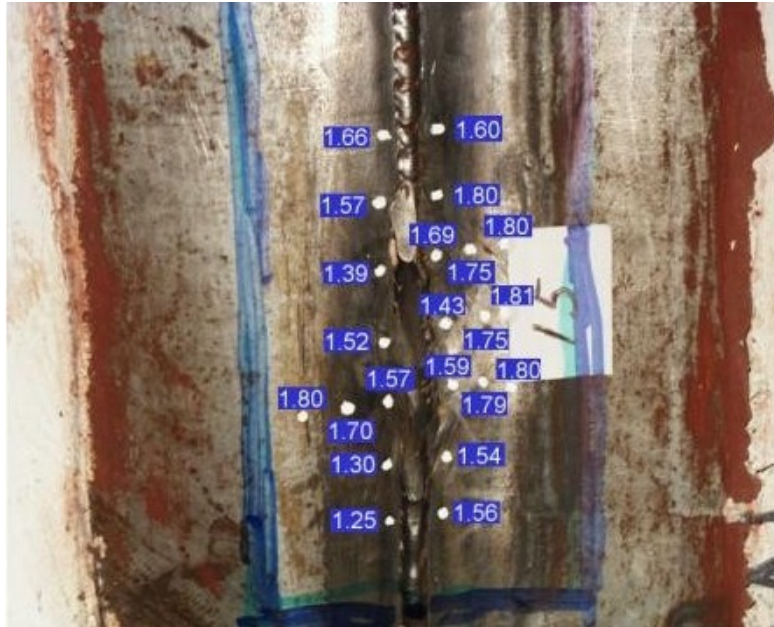
Figure 33. Liner thicknesses (in millimeters) measured ultrasonically in the vicinity of tear #15.
