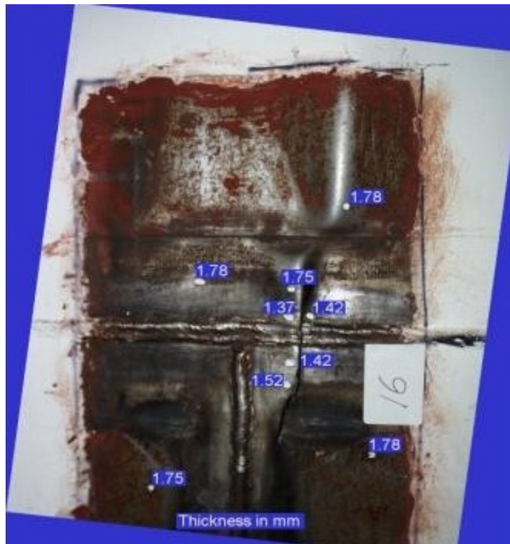
Figure 30. Liner thicknesses (in millimeters) measured ultrasonically in the vicinity of tear #16. Note distance of tear from vertical weld and extensive buckling above tear.
