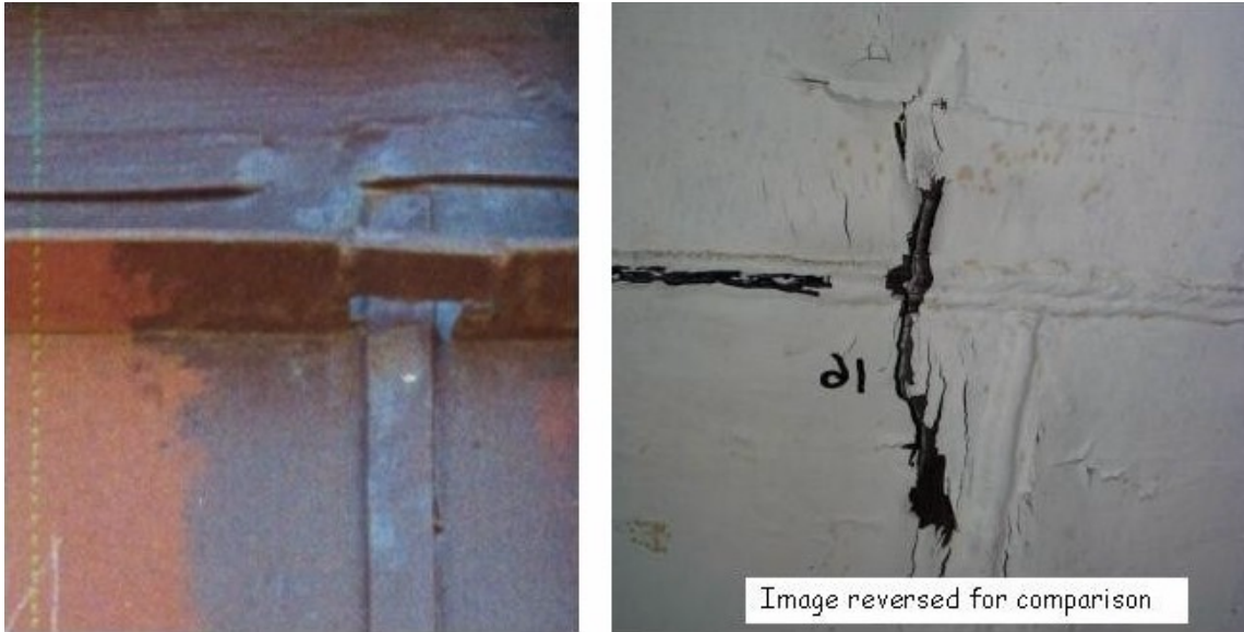
Figure 11. Photographs showing region of tear #16 from outside of liner (left) (prior to concrete placement) and inside of liner (right) (prior to removal of paint). Note missing segment of back-up bar on horizontal weld in vicinity tear.
