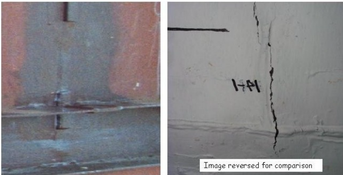
Figure 2. Photographs showing region of tear #1 from outside of liner (left) (prior to concrete placement) and inside of liner (right) (prior to removal of paint). The tear occurred under the wide segment of back-up bar near the top of the left-hand photograph, on the side closest to the anchor.
