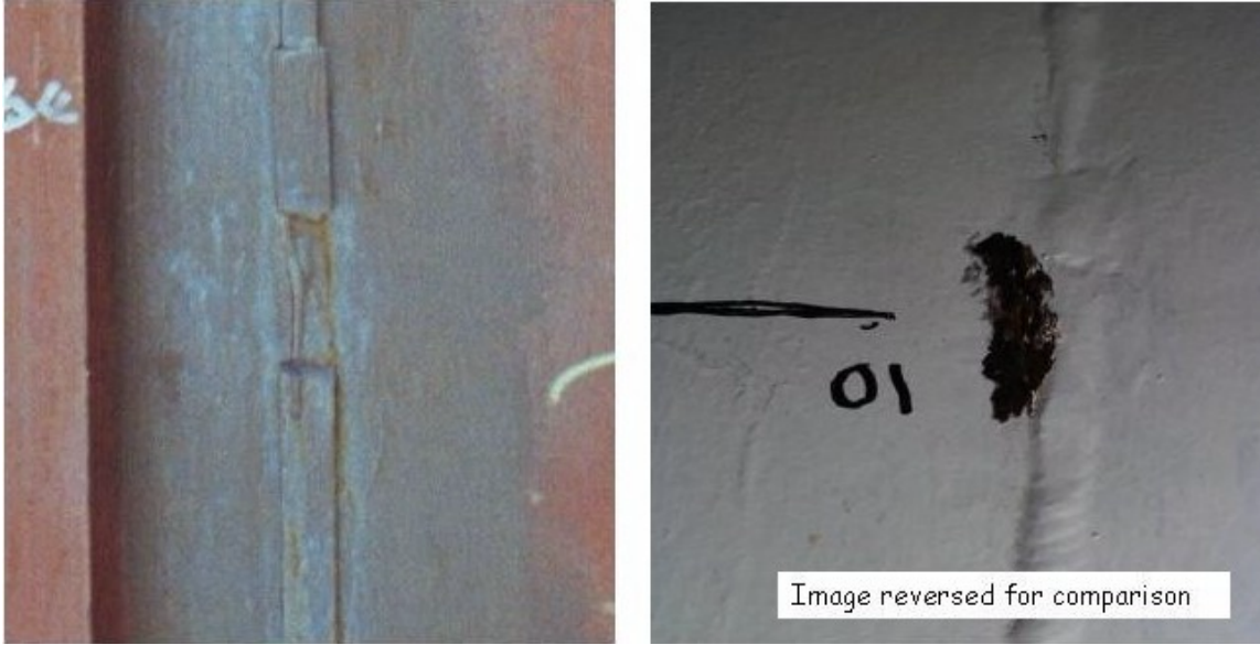
Figure 9. Photographs showing region of tear #10 from outside of liner (left) (prior to concrete placement) and inside of liner (right) (prior to removal of paint). Note missing segment of back-up bar in vicinity of repair weld and tear.
