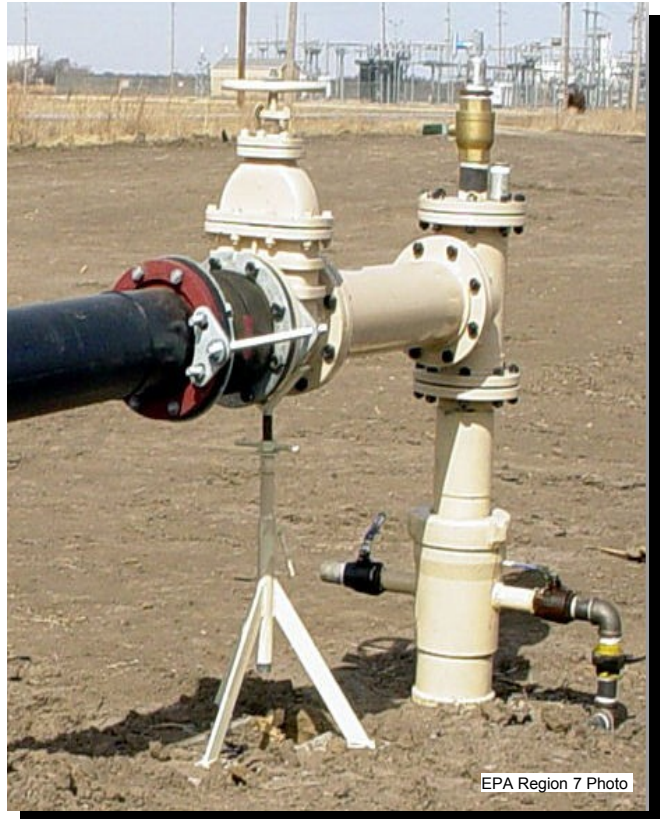
UNDERGROUND INJECTION CONTROL WELL HEAD
