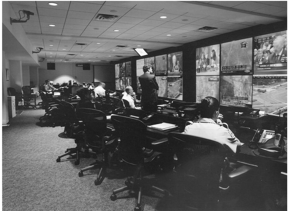
Figure 3: A CCTV Control Room
