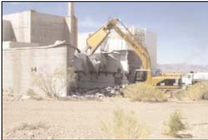
The Facilities and Infrastructure Recapitalization Program is on schedule and under budget thanks to innovative demolition techniques, such as the demolition processor (pictured above). This equipment allows for quicker demolition with a greater margin of safety.
