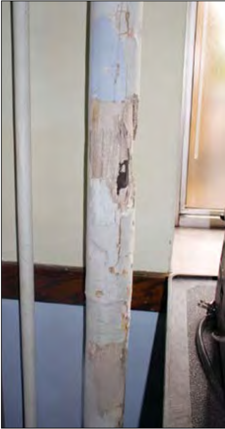
Deteriorating pipes can put students and staff in danger of falling debris and unknown contaminants.
