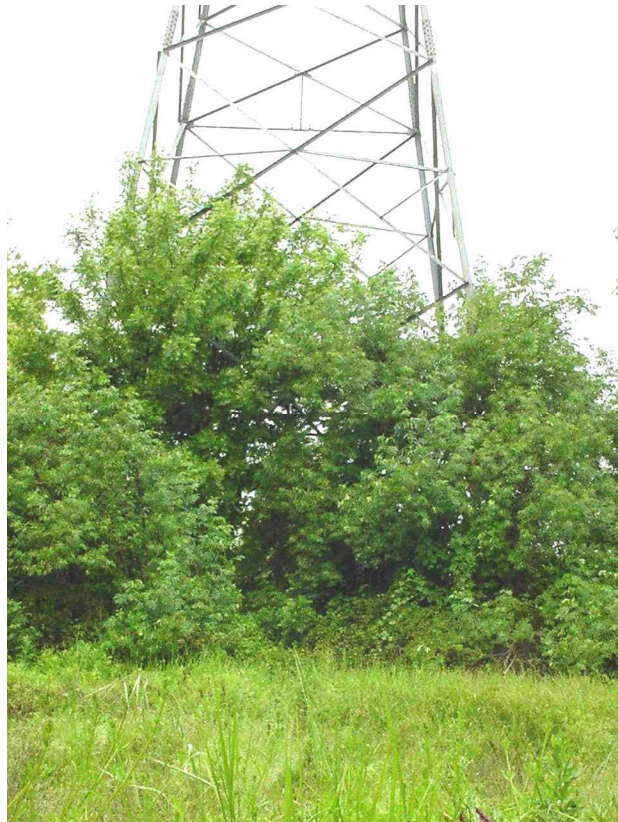
FIGURE 2-2. ELDERBERRY AND OTHER VEGETATION BLOCKING TOWER ACCESS
