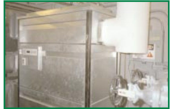
The Mariah CHP at Walker Court
