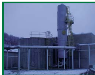
NATCO test site at Cedar Rapids wastewater treatment facility
