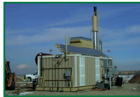
Quantum Leap Natural Gas Dehydration Technology (QLT) at a Colorado gas processing facility
