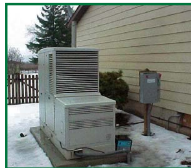
Power Plug field test site in New York
