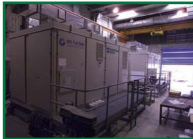
UTC fuel cells at wastewater treatment plant test site in Brooklyn
