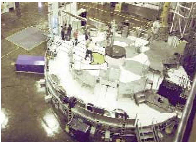
Reactor head, Advanced Test Reactor, Idaho National Laboratory
