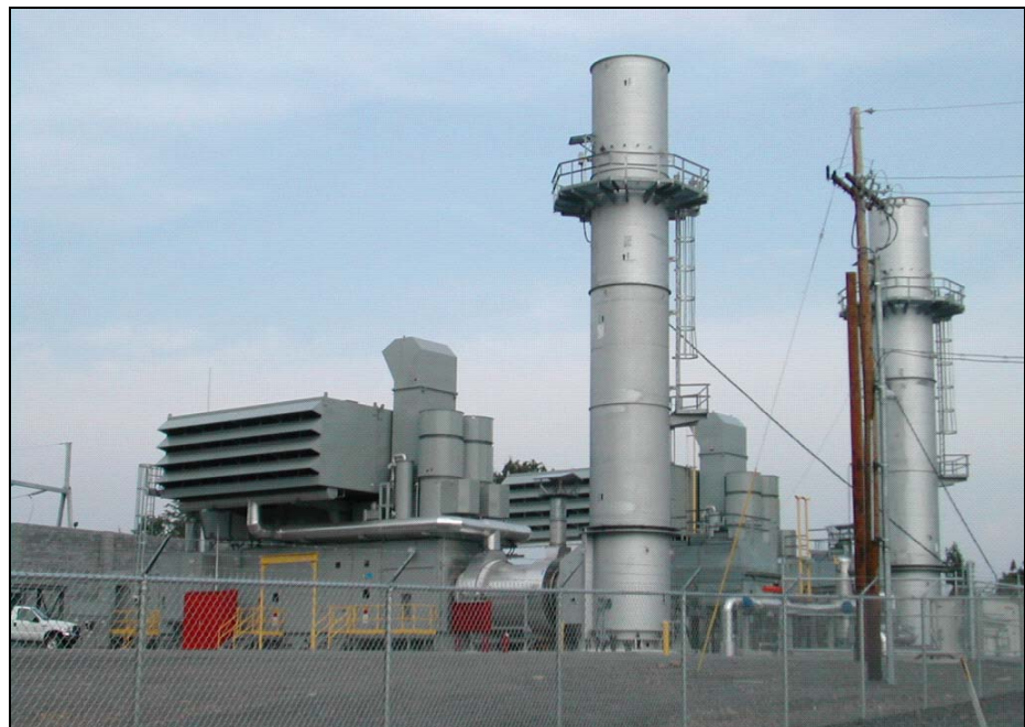
Consol Energy and Allegheny Energy's 88 MW Buchanan Generation Plant (photo courtesy of Consol Energy, Inc.)
