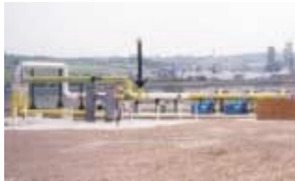
Alkane Energy's Markham Plant.
