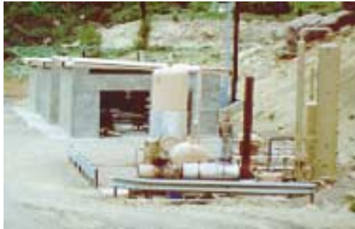
CMM collection and processing facility.
