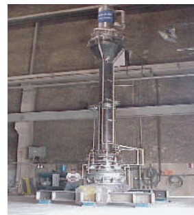
500 Gallon/Day TASHER LNG Plant. Photo courtesy of Appalachian-Pacific / Chart Industries.
