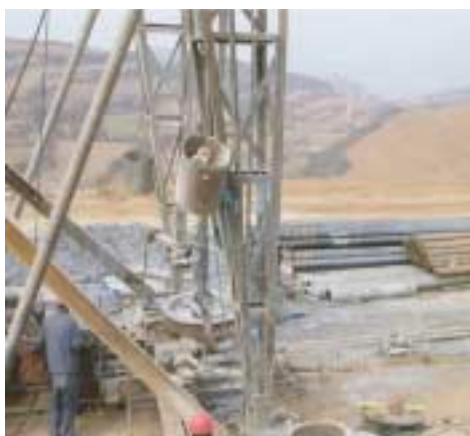
Drilling at Jincheng CMM Project, Shanxi Province, China. Photo Courtesy of ARI.
