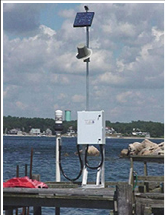
Water Level Station at Gray Gables, Massachusetts. The station, part of NOS's National Water Level Observation program, includes a data collection platform, acoustic sensor with a protective tube, satellite antenna, various meteorological sensors and solar panel to keep the battery charged.
