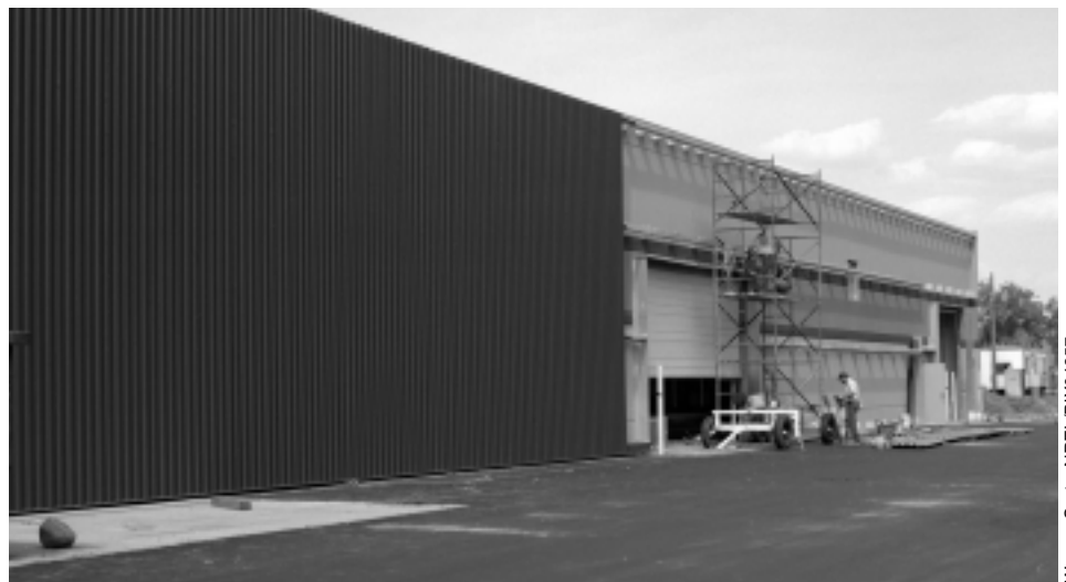
Figure 1. A transpired collector heating system being installed on a Federal Express facility in Littleton, Colorado.
