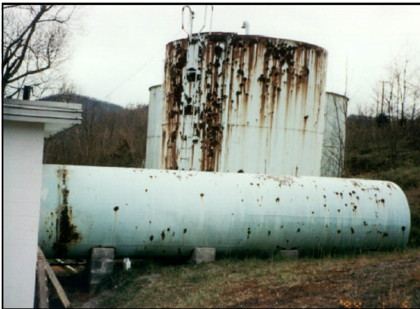
The rust on the hydropneumatic tank (foreground) signals the need for rehabilitation, while the severe corrosion on the other tank will require its replacement. Such deterioration can promote microbial growth and impair water quality.
