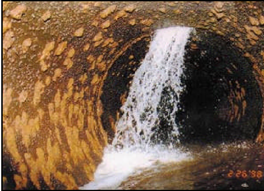
Water from the Charles River in Massachusetts pours into a deteriorated transmission main which the Massachusetts Water Resources Authority (MWRA) had drained after detecting a leak. MWRA replaces or rehabilitates approximately 7 miles of pipe per year, some of which is more than 100 years old. Many older water systems will find it increasingly necessary to replace substantial portions of distribution networks that were installed 50 to 100 years ago.
