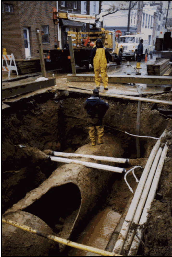
Workers repair a water main break in Philadelphia. Deteriorated distribution pipe is susceptible to microbiological contamination and can disrupt water service.
