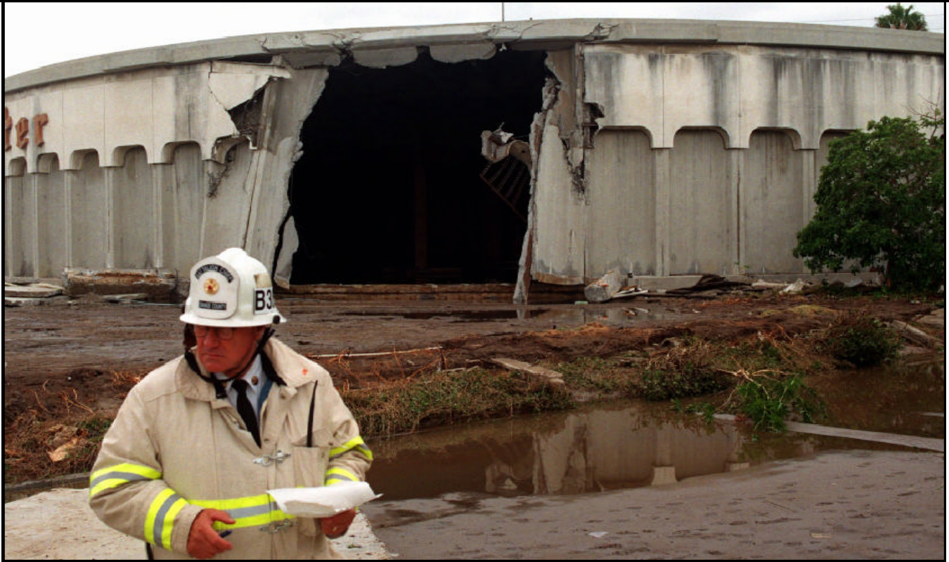
This 31-year-old storage tank ruptured in Westminster, California, sending a 6-foot wave of water through the city that damaged or destroyed about 50 buildings and over a dozen vehicles. Storage tanks should be replaced or periodically rehabilitated to preserve their structural integrity.
