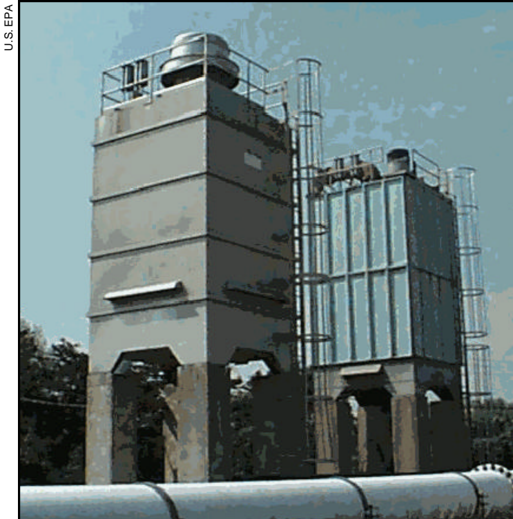
Water systems use a variety of treatment technologies to remove harmful contaminants from drinking water. For example, aeration units (pictured) are used to remove volatile organic compounds and certain secondary contaminants, such as hydrogen sulfide.
