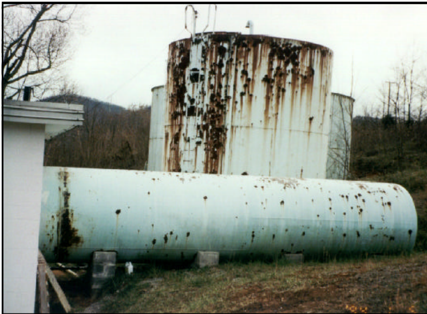
The rust on the hydropneumatic tank (foreground) signals the need for rehabilitation, while the severe corrosion on the other tank will require its replacement. Such deterioration can promote microbial growth and impair water quality.
