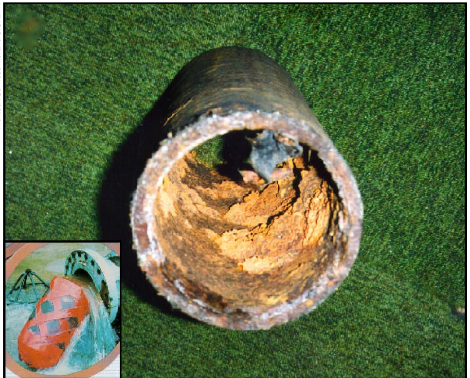
This pipe shows clear signs of tuberculation, a condition resulting from the accumulation of mineral deposits and debris. Tuberculation can reduce pipe capacity and impair drinking water quality. One method of removing tubercles involves sending a “pig” (insert) through the system to scour the sides of the pipe.
