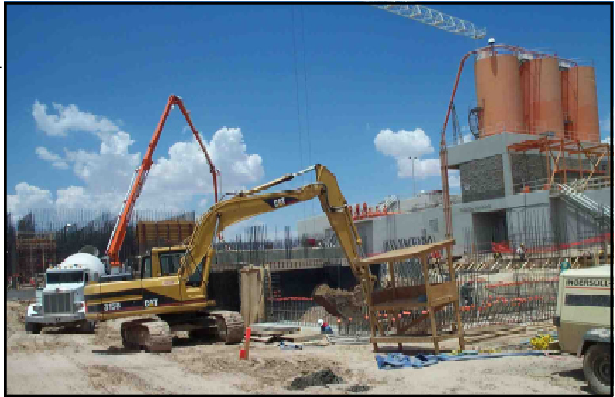
The City of El Paso, Texas, received a $15 million loan from the Texas DWSRF program to expand the capacity of the Jonathan Rogers Treatment Plant. This project will provide water to colonias that lack access to safe drinking water.
