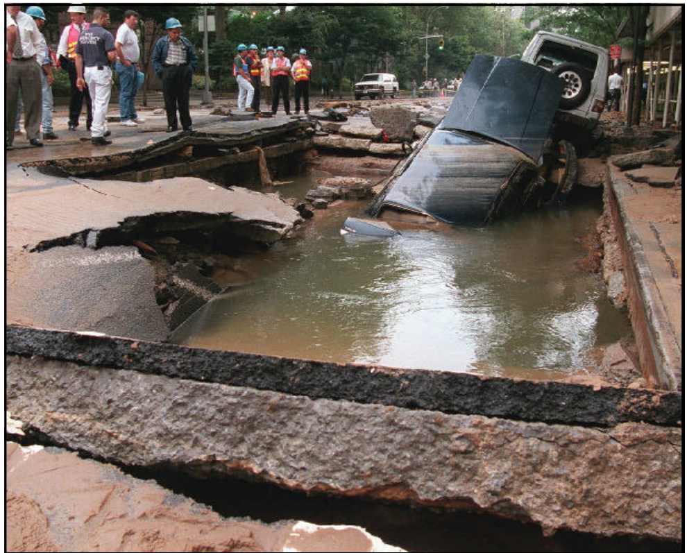
A ruptured water main in New York City closed a section of a major thoroughfare and limited service to two hospitals. The majority of the nation's distribution lines were installed in the mid-1900s. Towns and cities are finding it increasingly necessary to replace old and deteriorated pipe.
