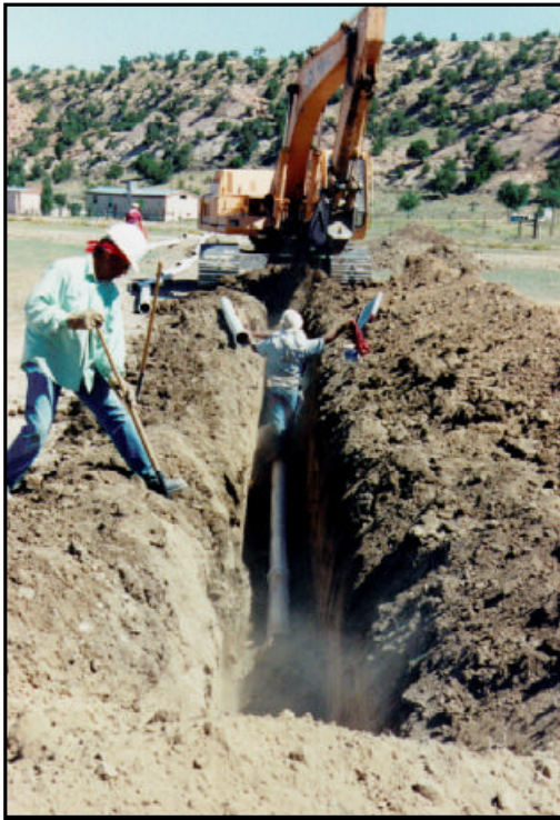
Workers install a section of water main on the Navajo reservation in Arizona. Many American Indian systems have disproportionately high distribution needs relative to their size, because they serve widely dispersed homes in remote locations.
