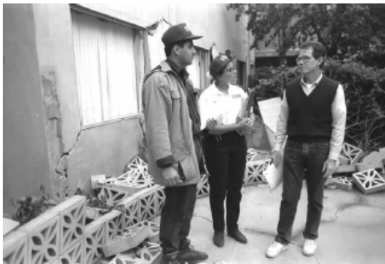
A trained inspector makes an on-site assessment of damage on behalf of the State-administered Individual and Family Grant Program and FEMA's Disaster Housing Program.
